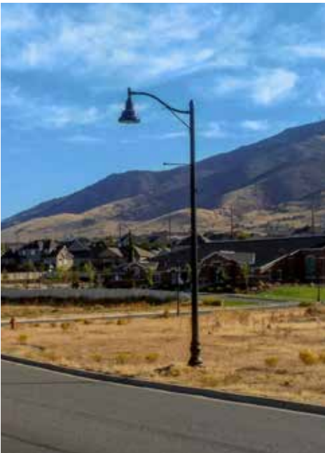
20' Collector Street Light
